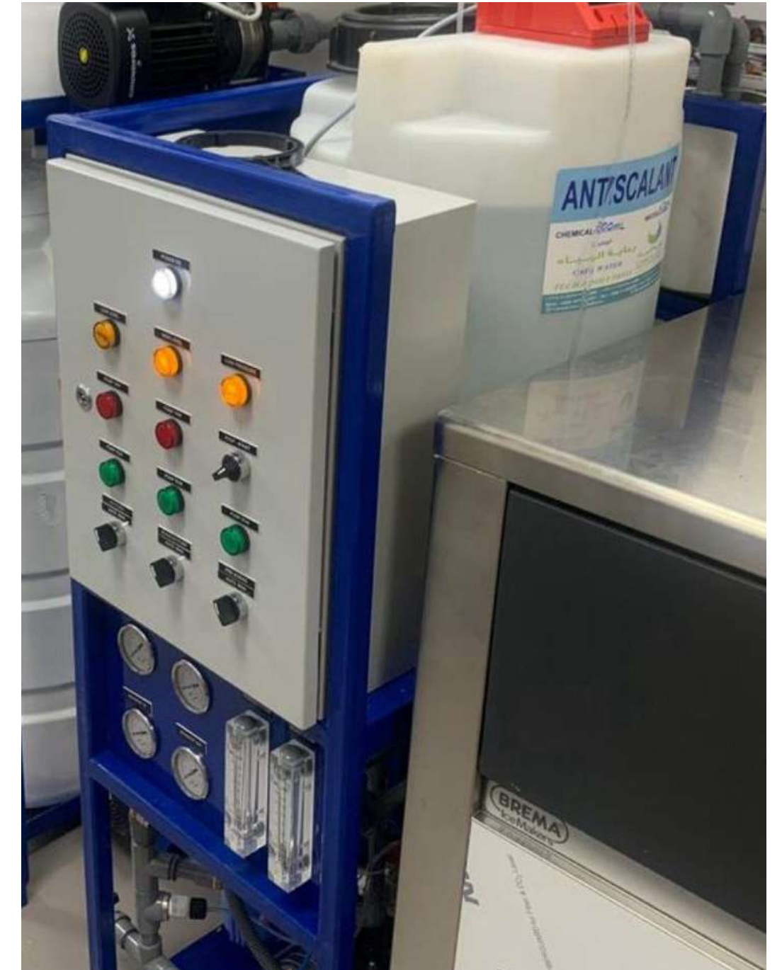
Reverse osmosis system
